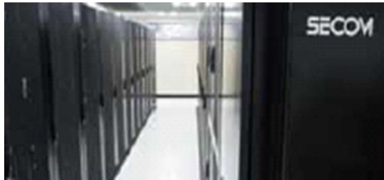
Secure Data Center Service
