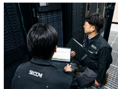
Inside the Secure Data Center® TC4
