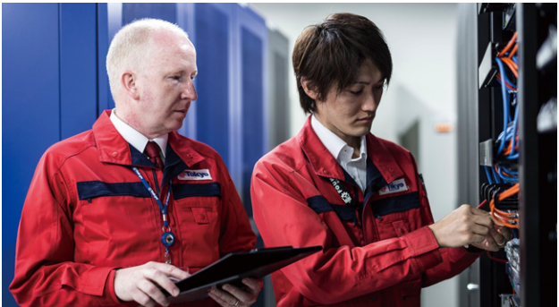
At Tokyo data center
