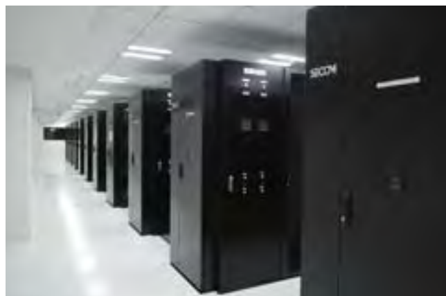
Secure Data Center
