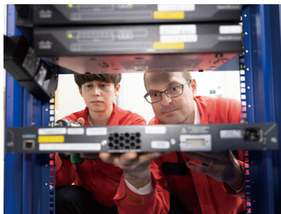
At Tokyo data center
