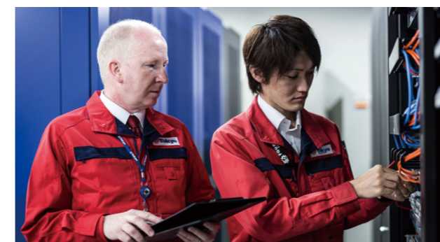
At Tokyo data center
