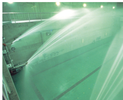
Test of fire extinguishing system (Nohmi Bosai)
