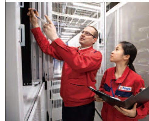
At Tokyo data center
