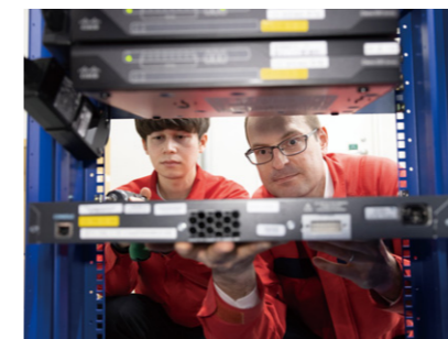
At Tokyo data center
