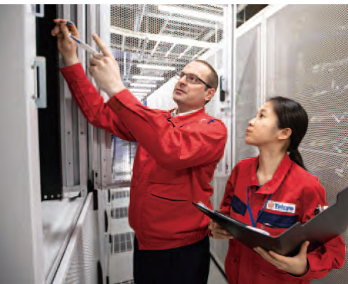
At Tokyo data center
