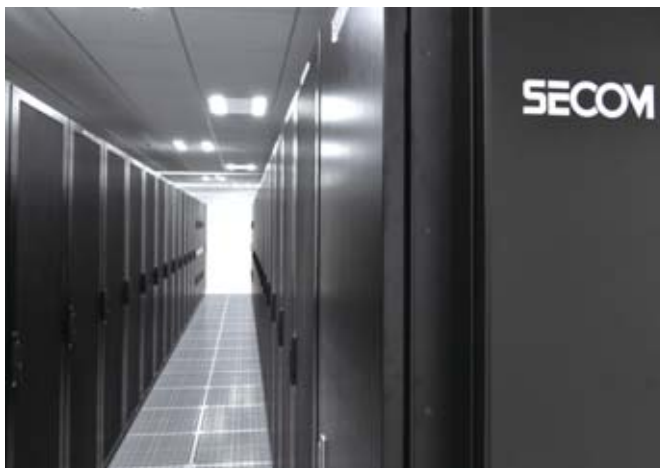
SECOM data center facility
